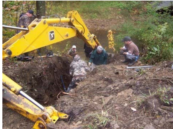
Construction of a streambank stabilization structure on Kratzer Run, a tributary to Anderson Creek. Photo courtesy Malcolm Barnes.
