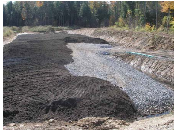
Vertical flow pond at the Glasgow site, during final placement of new compost over limestone. Photo courtesy Arthur Rose.
