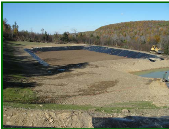
Klondike KL-2 Treatment System
